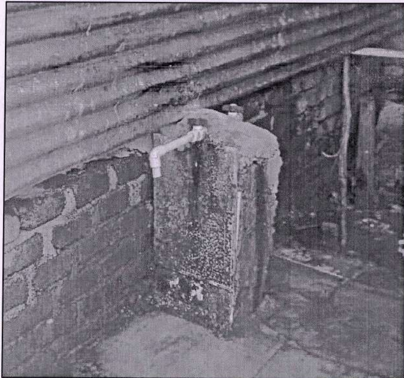
Drinking Water Supply
